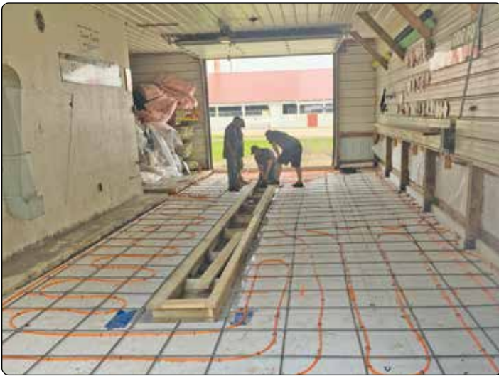
The new floor on the groomer half of the Driftrunners clubhouse includes a center trough drain, insulation and tubing for in-floor heating in the future.
